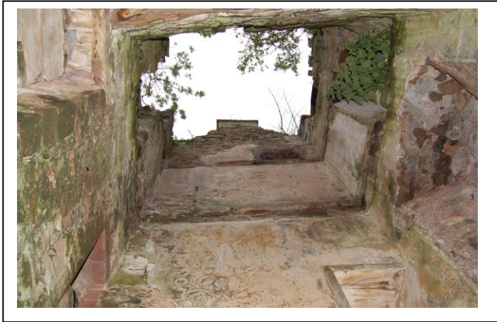
Fig. 22: Left: View up inside the east tower from the ground floor. Shelley 2008.
